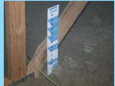
An insufficient amount of insulation in the attic was contributing to the Stuemkes' home energy problems. "They started with about 3½ to 4 inches of insulation, which is about one-fourth of what they should have up there," says Zurliene.
