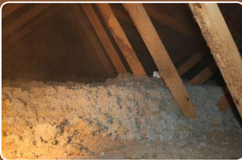
The view attic after sufficient insulation had been installed. "The U.S. Department of Energy recommends insulating to an R-49 value, which with our product, translates to a thickness of 15 inches," explains Zurliene. "You can see quite a difference in elevation from what it looked like before."
