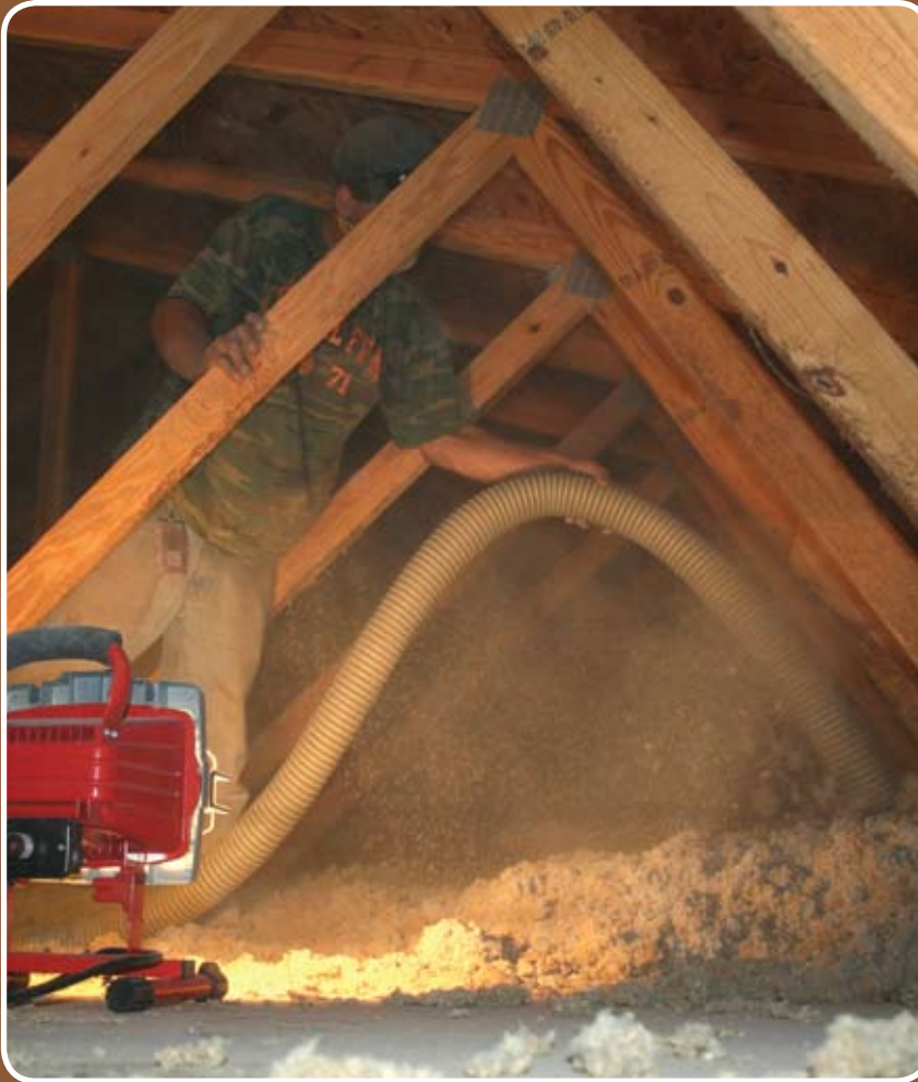
Dave Hall, a Spray Insulation & Contracting employee, installs high-density, loose-fill cellulose insulation in the attic. Their product is effective at resisting heat and cold ranging from -21 to 121 degrees Fahrenheit.
