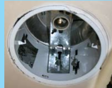
Air leaks are also common in recessed can lights. These fixtures had additional openings for screws, which Spray Insulation employees closed off with heat-resistant metal tape. "Heat radiating off the light bulb creates what we call a 'chimney effect' where hot air is forced out of the screw holes and replaced by unconditioned air from the attic," explains Zurliene.
