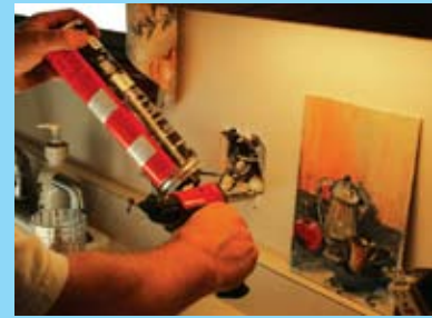
"Light switch and outlet receptacles are notorious spots for air leaks," says Zurliene. "So we applied foam sealant behind the outlet and switch boxes."
