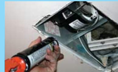
The contractors applied caulk around the edges of exhaust fans to reduce the air flow coming in from the attic.
